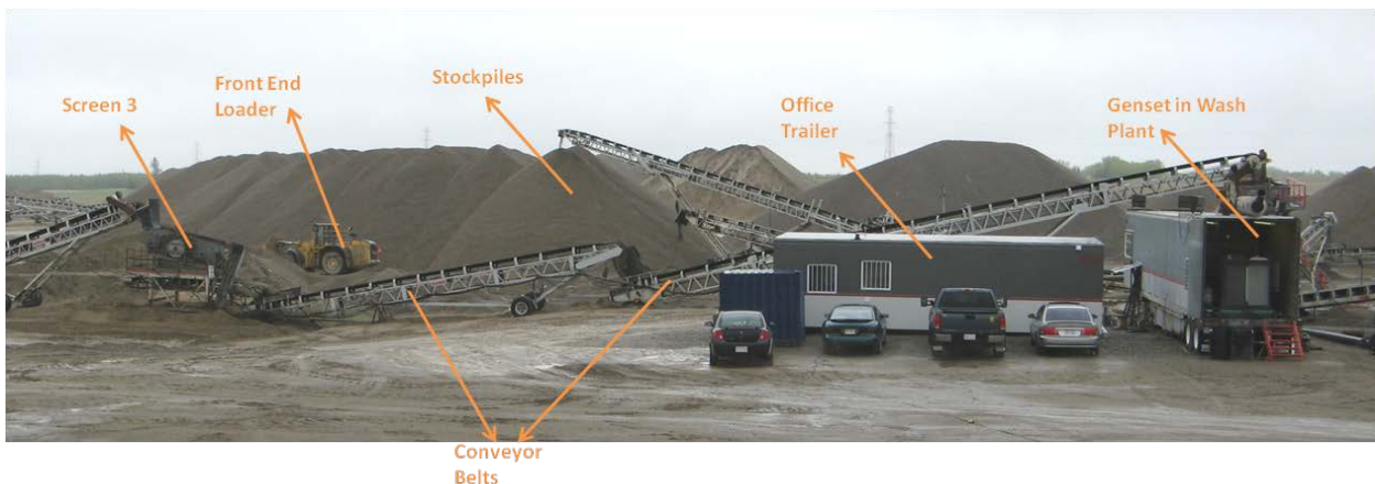
Photo 2: Some of the Equipment Associated with the Wash Plant
