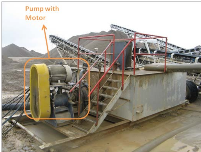
Photo 13: Washer Pump with Motor in the Wash Plant
