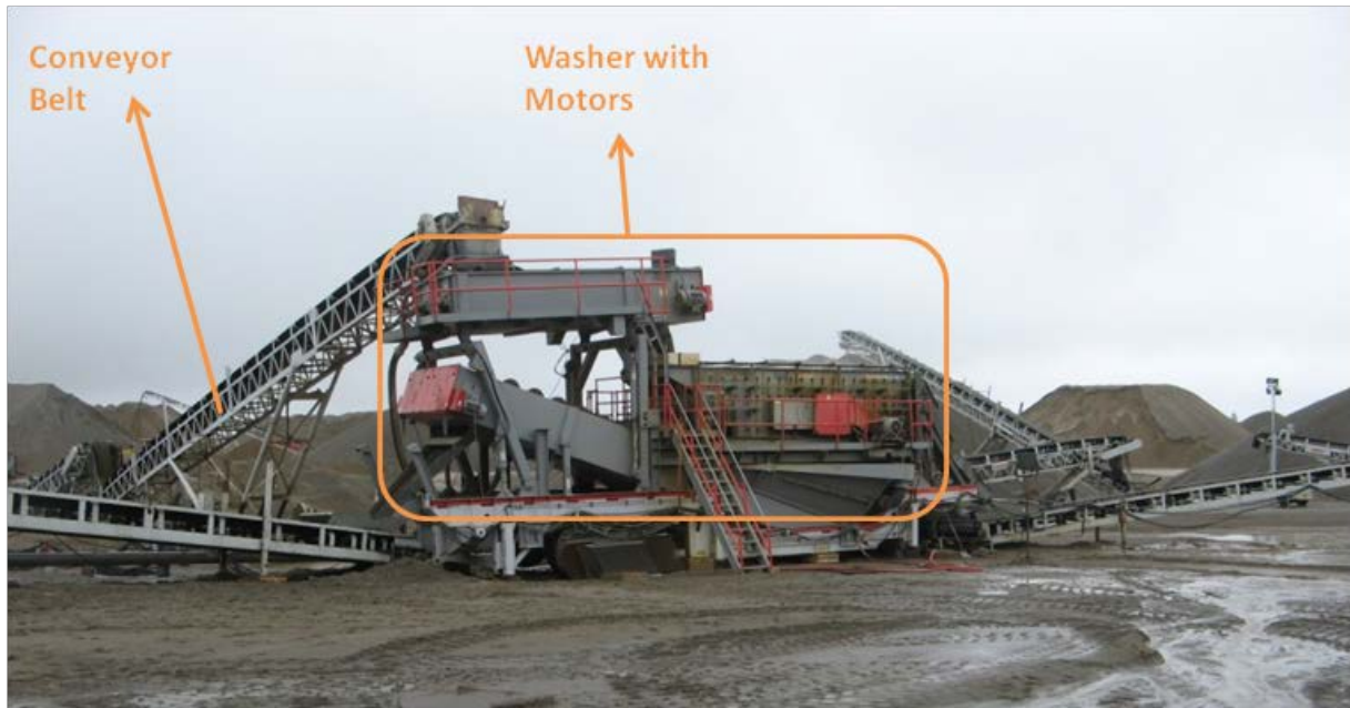
Photo 12: Washer Unit in the Wash Plant
